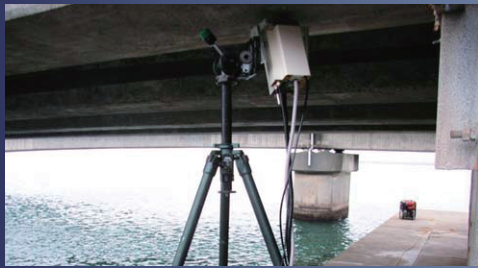
Analysis of the surface of bridge pier
